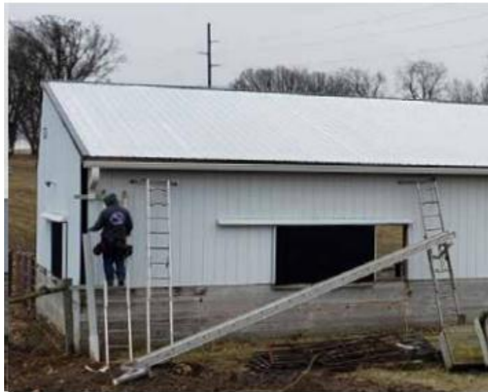
AFTER - Installing roof gutters at the Laeser property. Photo courtesy of Iowa County
