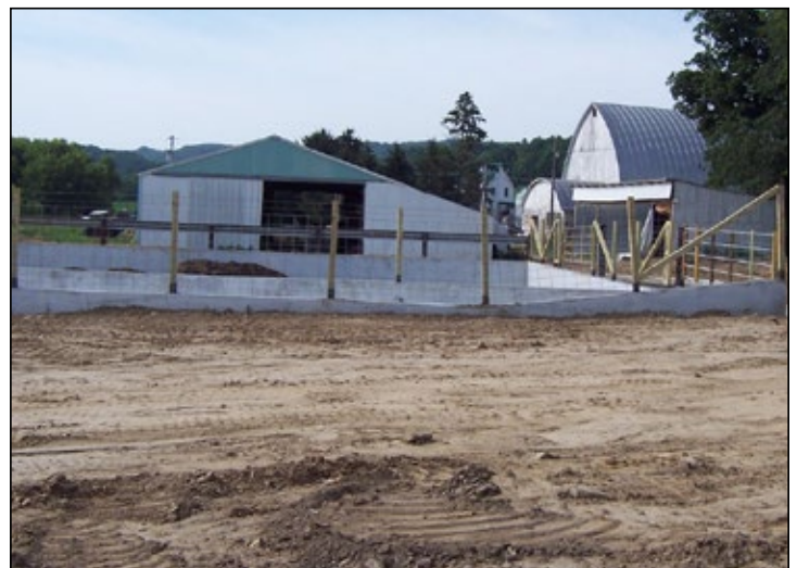
Completed manure storage structure in Monroe County partially funded with a cost-share grant
