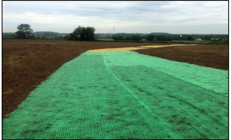
An installed grassed waterway system with erosion control netting and a turf reinforcement mat in Fond du Lac County
