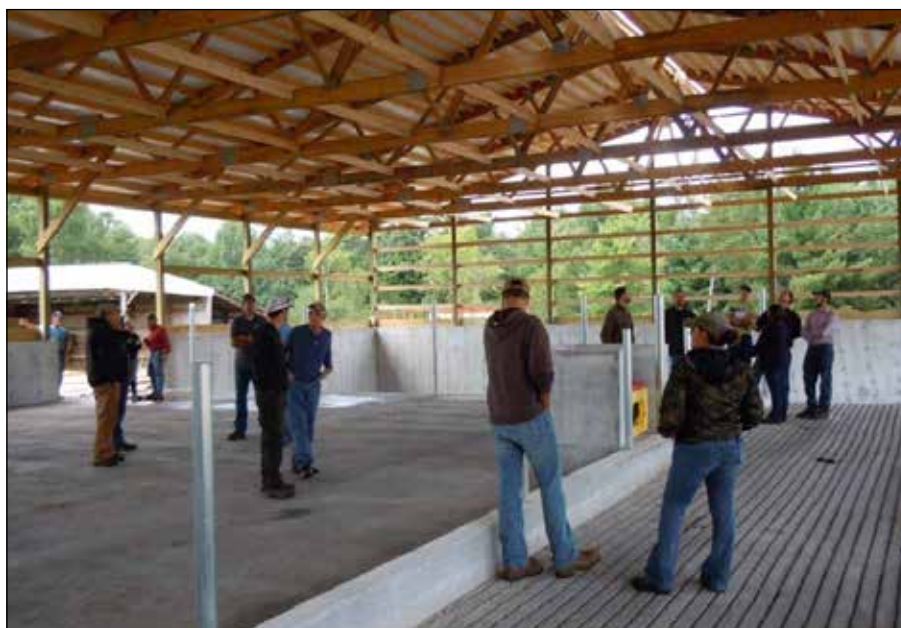
A roofed winter feedlot project provided a training opportunity for staff from conservation agencies in northwest Wisconsin. Photo: Burnett County Land Services Department
