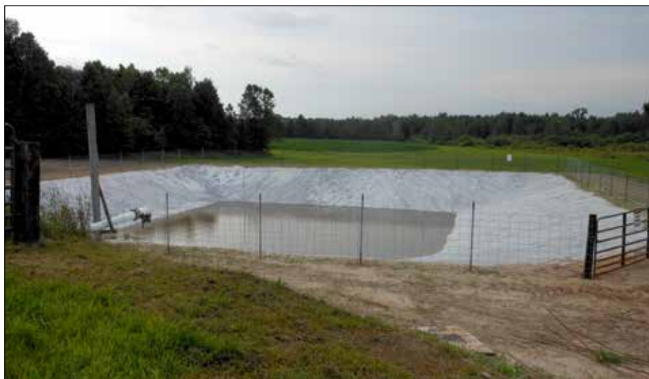
A manure storage facility. Photo: Rusk County Land and Water Conservation Department
