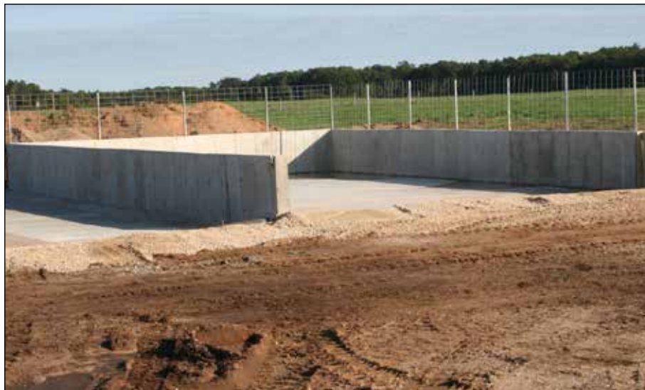
A manure stacking facility allows liquid from manure to drain off for pumping, with dry manure left in storage. Photo: Waushara County land Conservation Department
